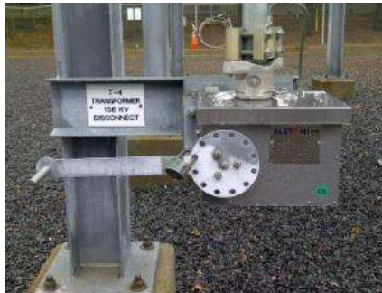
Disconnect switch manual mechanism
