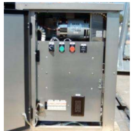
Disconnect switch motor operator
