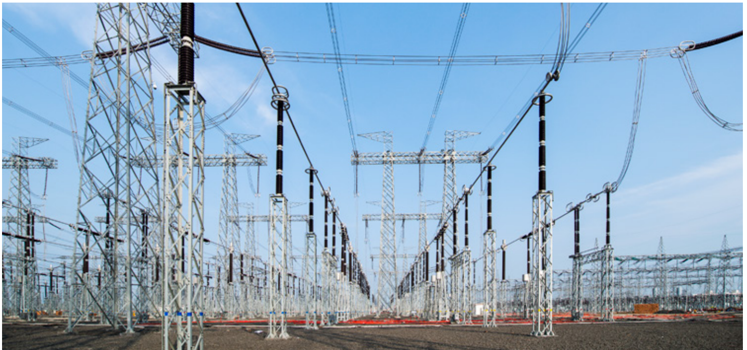
HVDC Substation Bina, India
