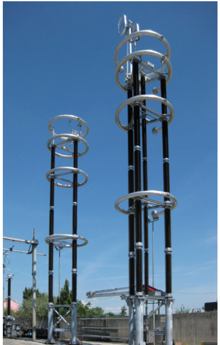
Outdoor Testing for Disconnectors
