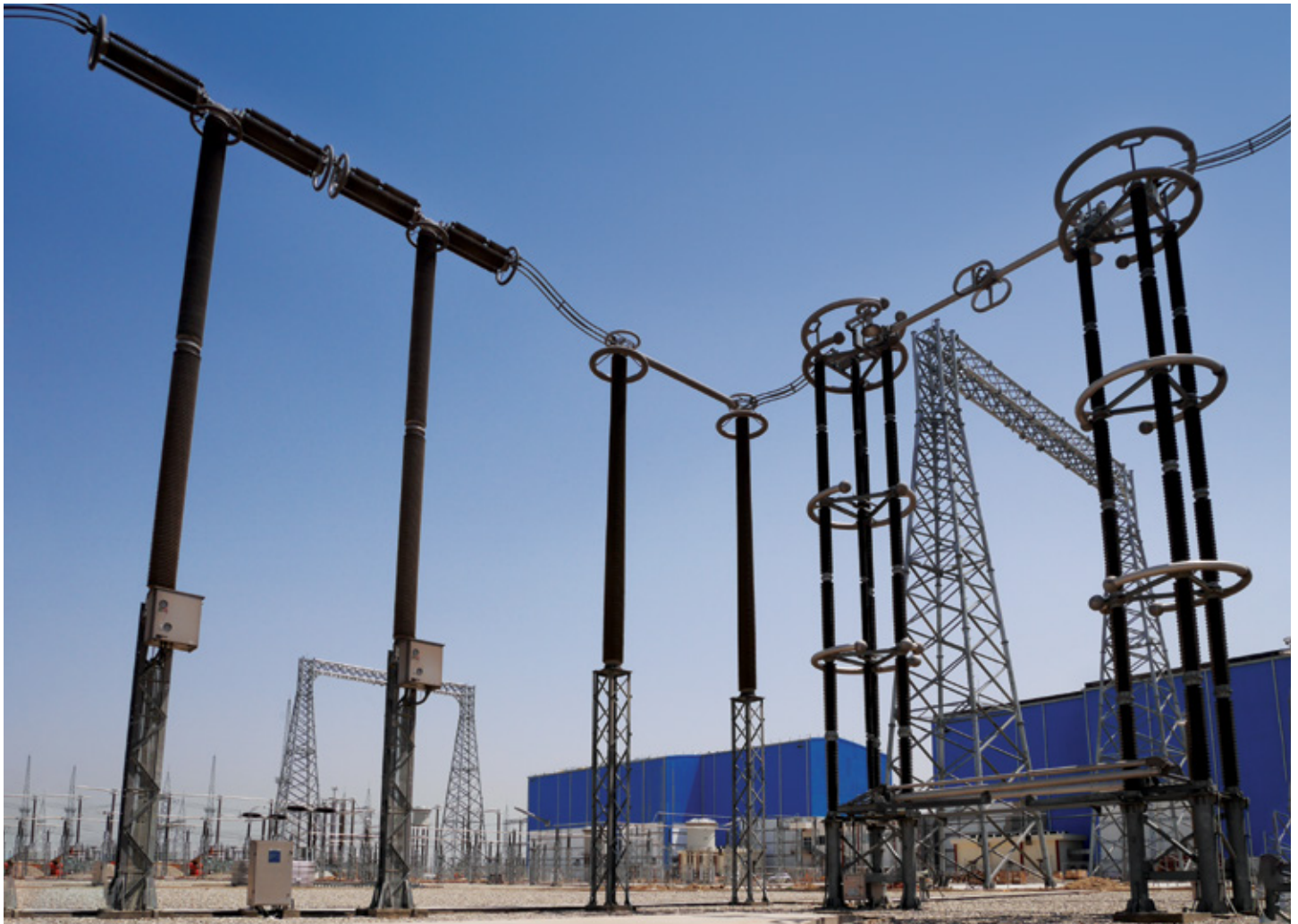
HVDC Substation Bina, India
