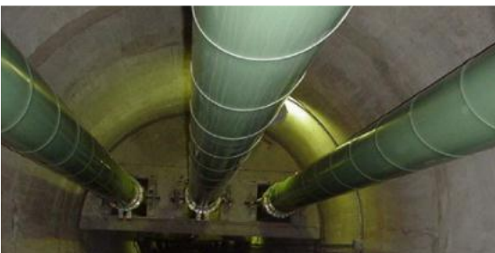
362 kV GIL in vertical shaft (140 m high) Total length: 900 m
