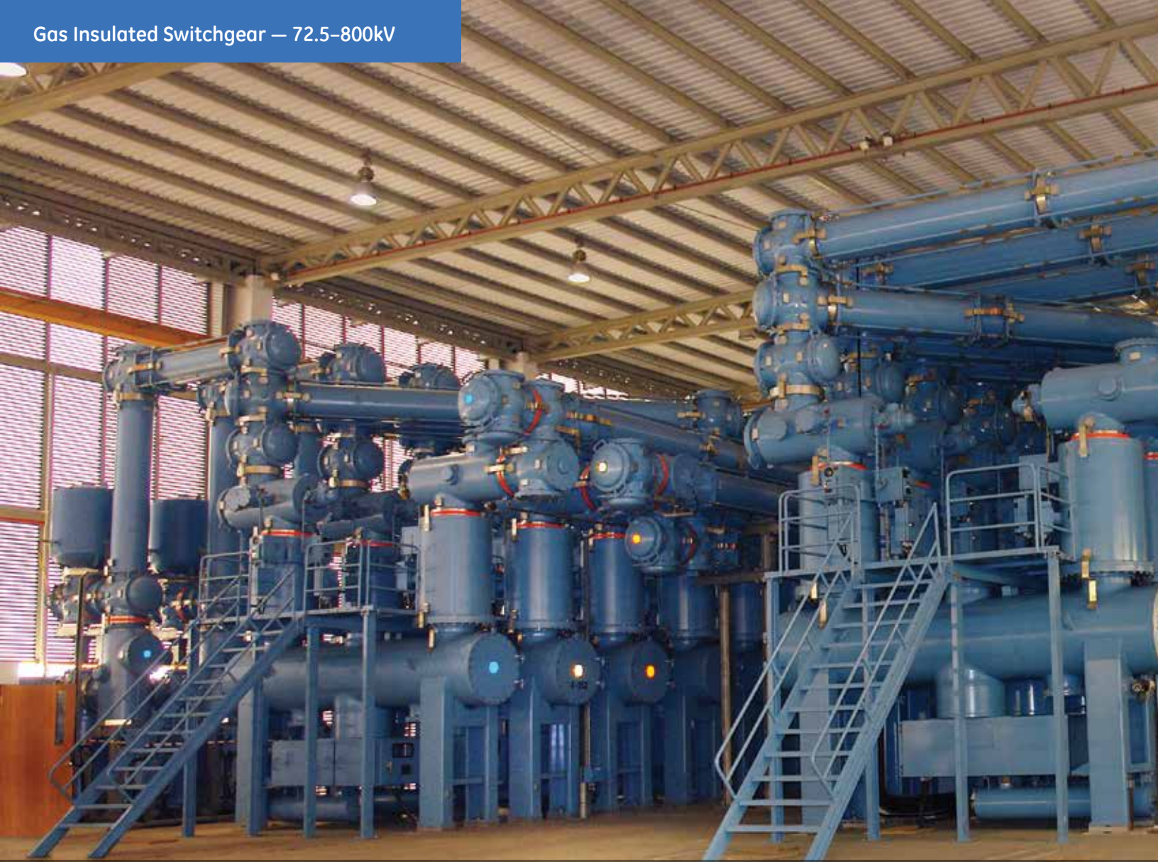
420kV Gas Insulated Switchgear
