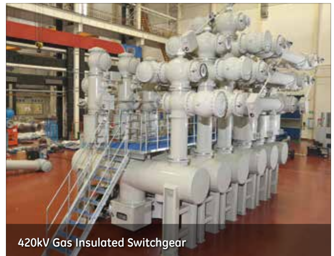
420kV Gas Insulated Switchgear
