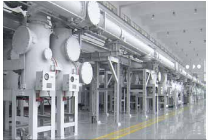
550kV Gas Insulated Switchgear
