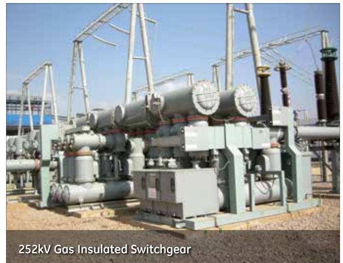
252kV Gas Insulated Switchgear
