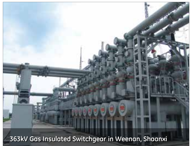
363kV Gas Insulated Switchgear
