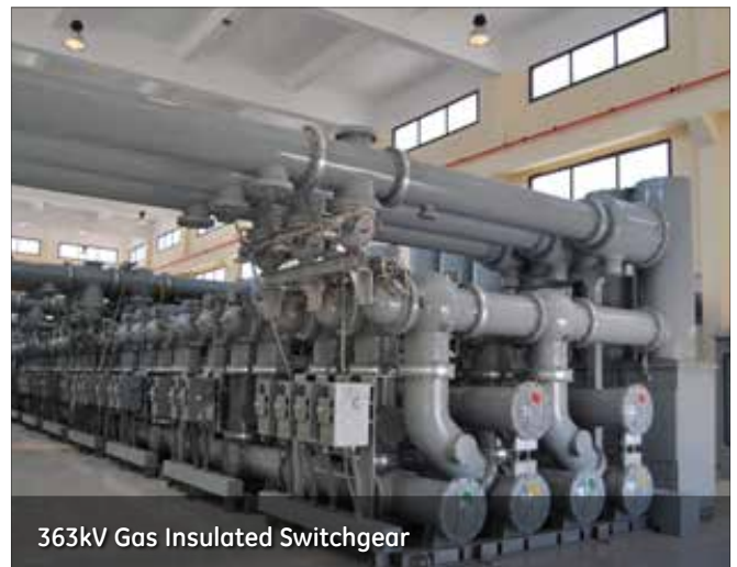
363kV Gas Insulated Switchgear at Golmud Substation
