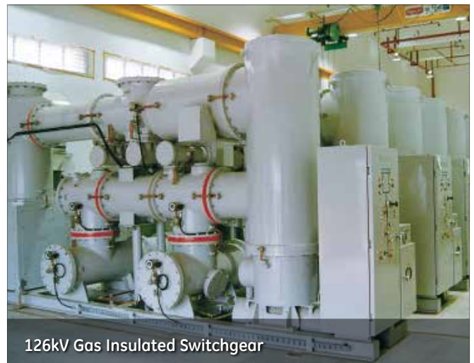
126kV Gas Insulated Switchgear
