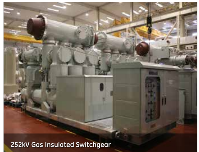
252kV Gas Insulated Switchgear
