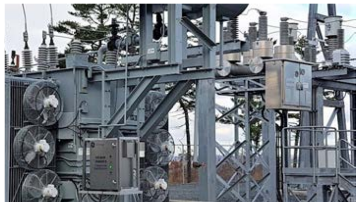
20MVA transformer with Transfix DGA monitor
