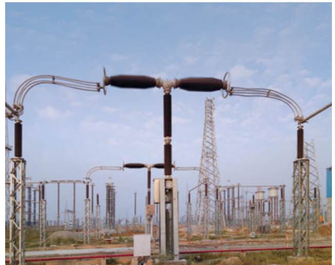
DC Switch in Champa India
