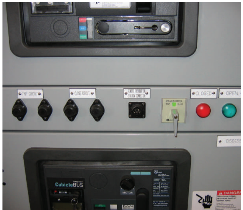
Control port on WL Switchgear
