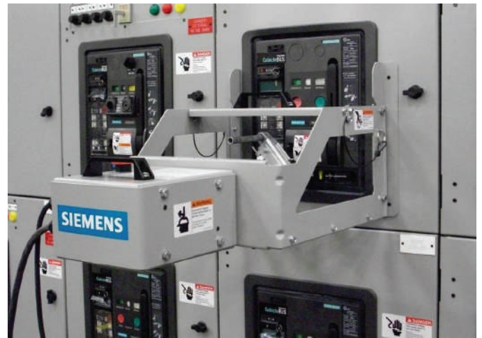
Remote Racking Device
