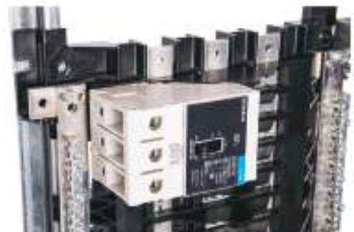
Example of Back-fed NGB Main breaker installed
