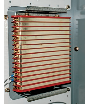
Figure 34: Secondary disconnect cell portion
