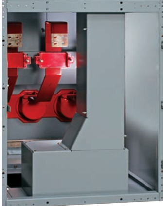
Figure 9: Cable trough in lower cable compartment to isolate cables from circuit breaker in upper compartment
