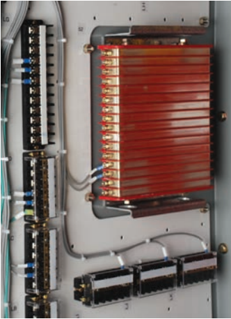
Figure 20: Circuit breaker cell wiring and secondary disconnects
