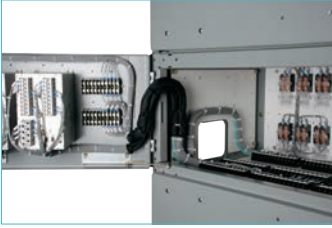
Figure 19: Protective relay and instrument cell interior
