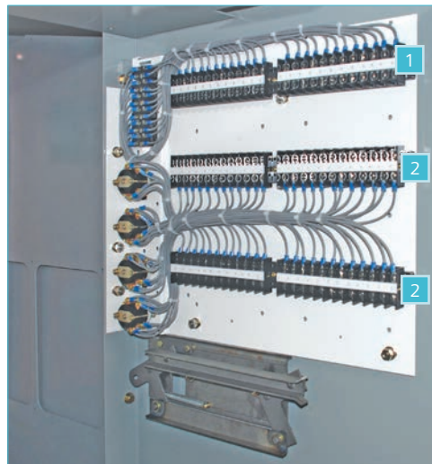
Figure 36: MOCs and TOCs (cover removed)
