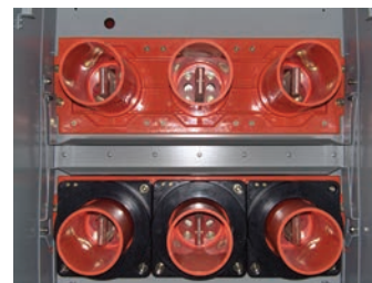
Figure 13: Type MD CTs installed on lower disconnect bushings (CT barrier removed for photo)
