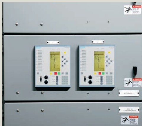
Figure 28: Type GM-SG protective relay and instrument compartment
