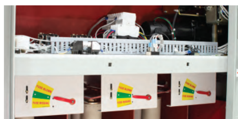
Blown fuse window with indication flags and motor-operated switch, shown with main door open
